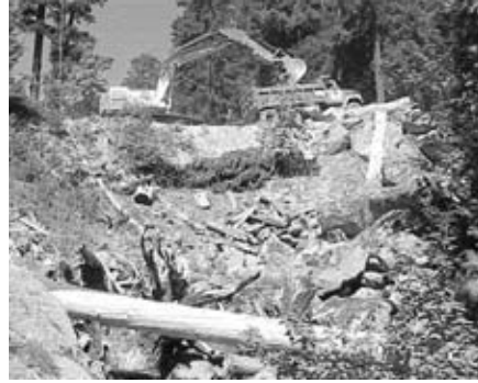
Major road fill before removal. Road restoration activities, especially decommissioning, stabilization, and fish passage, are a major element of the Restoration Program and account for nearly 60% of annual restoration funding.
