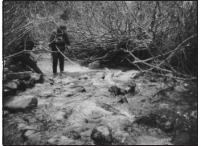
Figure 2. After the fine material had been loosened, it allowed the boulder to be excavated and used in constructing the riffle structure.
