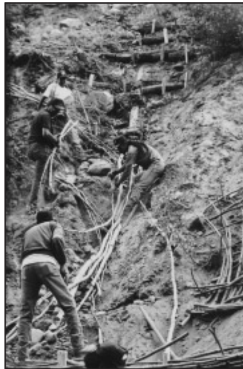
Figure 2. Boston Bar participants building a live pole drain as part of their bioengineering training.
