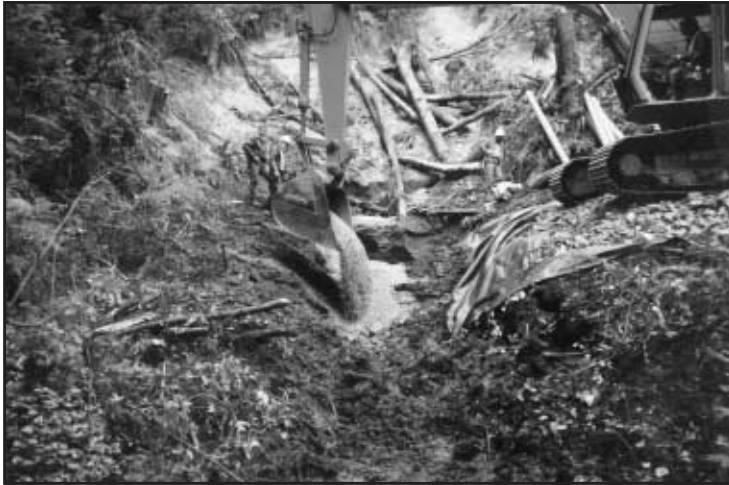
Figure 2. Slope failure in Kendale Creek ravine, North Delta, BC.
