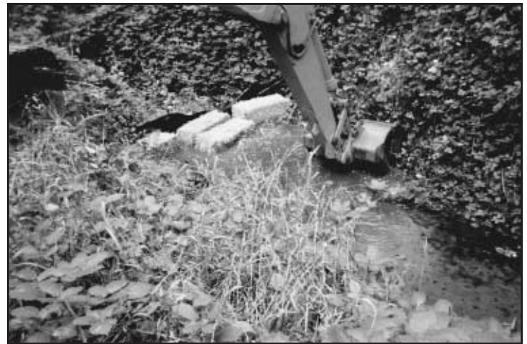
Figure 7. Restoration of Pool 3 showing placement of rip rap to stabilize undercut banks and of LWD to increase rearing habitat.
