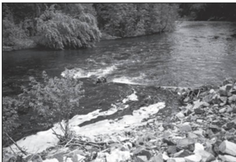
Figure 4. An example of a box groin designed to maintain pool habitat for trout and whitefish at a logged section of the West Kettle River.
