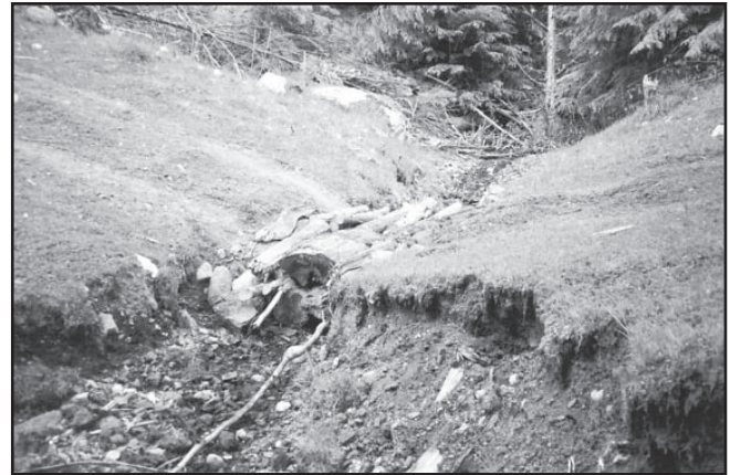
Figure 3. This stream restoration should have allowed for vehicle access, but the lack of adequate armouring resulted in the down-cutting of the stream channel. To regain access, a salvage crew has placed logs into the structure. Note, also, that the vehicles have scraped off the protective layer of grass on both approaches, which will further exacerbate the sediment problem.
