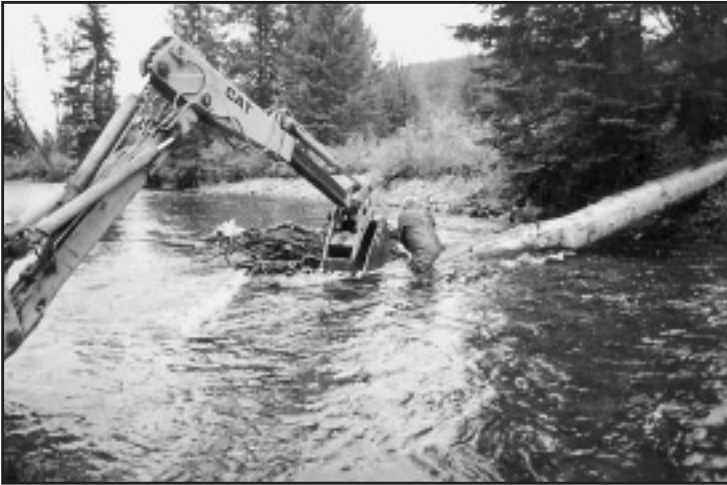
Figure 3. The construction of a lateral log jam in 1996. Note the shallow water.
