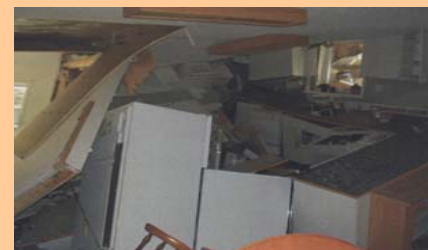
Damaged House: Kuskonook Creek Slide
