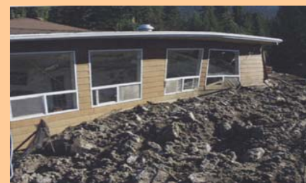
Damaged House: Kuskonook Creek Slide
